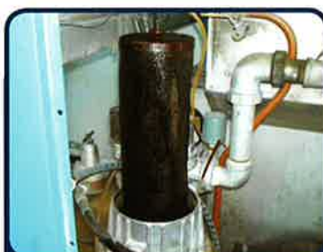
Oil separator abnormal clog
